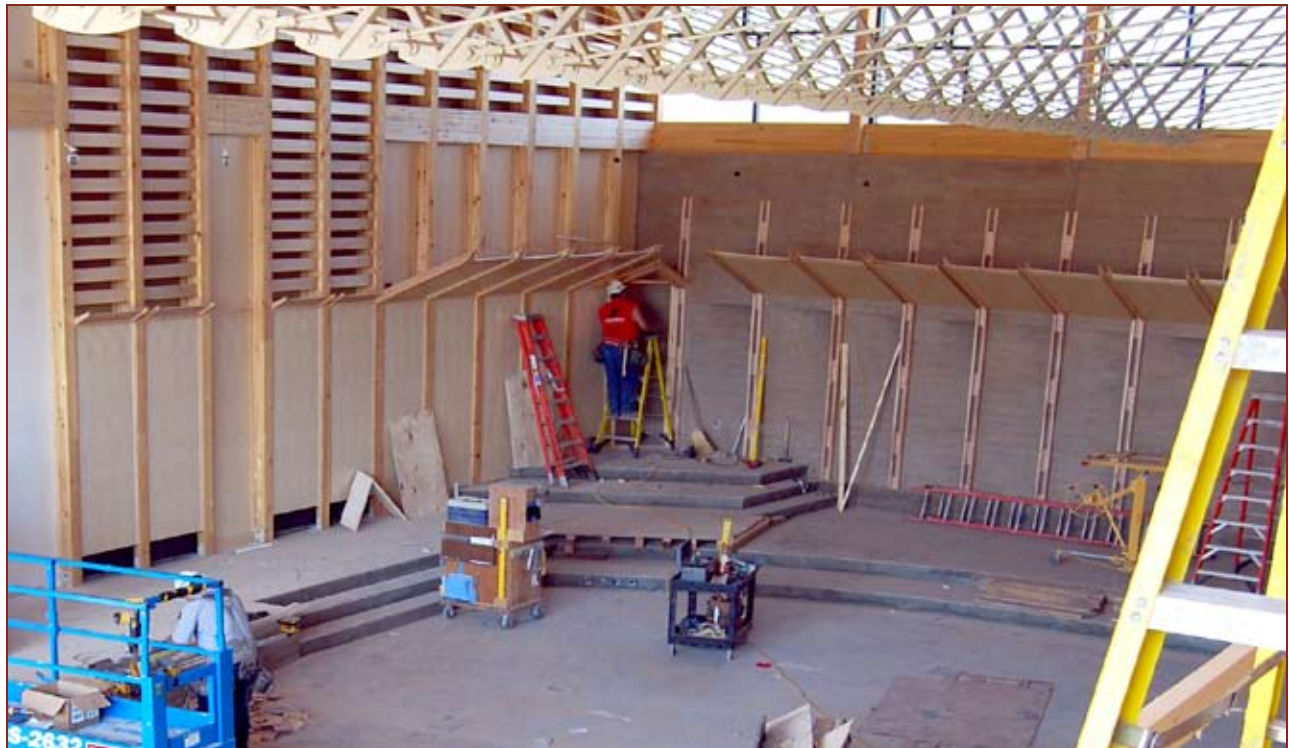
Finish work continues in the Auditorium as AV equipment, lighting, painting and woodwork are all being completed.
